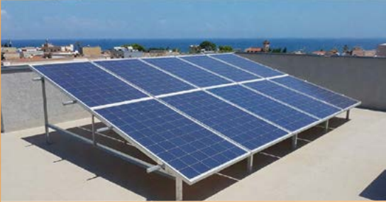
SOLAR POWER PANELS
